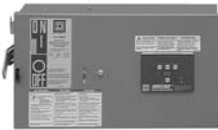
Busway SURGELOGIC TVSS Unit
