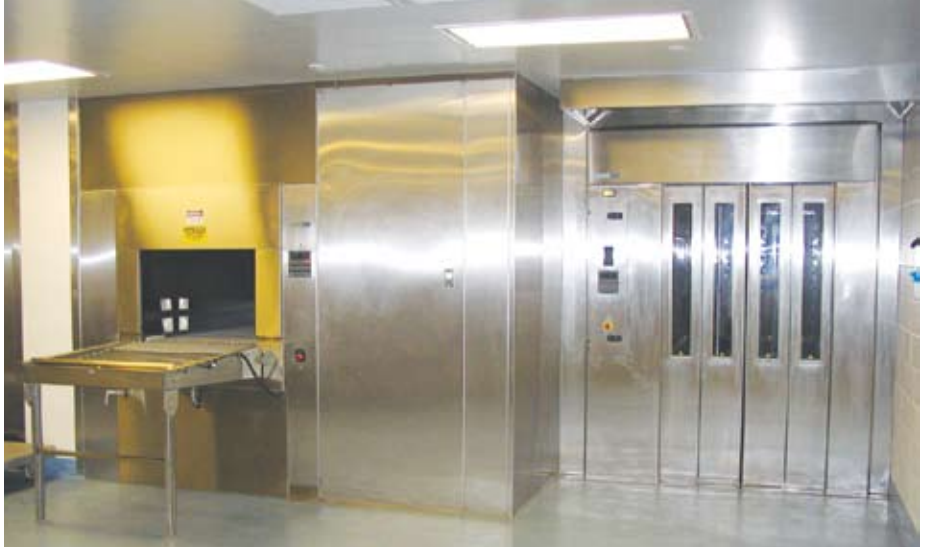
Moffitt Vivarium Tunnel Wash System
