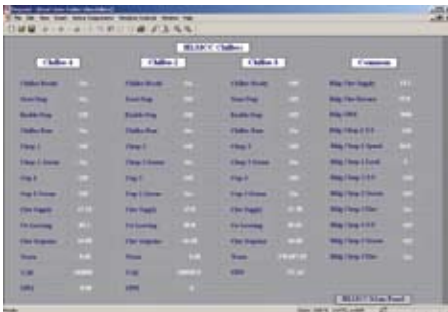
A CyberStation™ Chiller Status Screen
