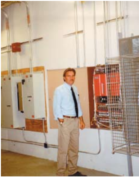
Dean Head, Moffitt's Director of Facilities, inspects some TAC controllers
